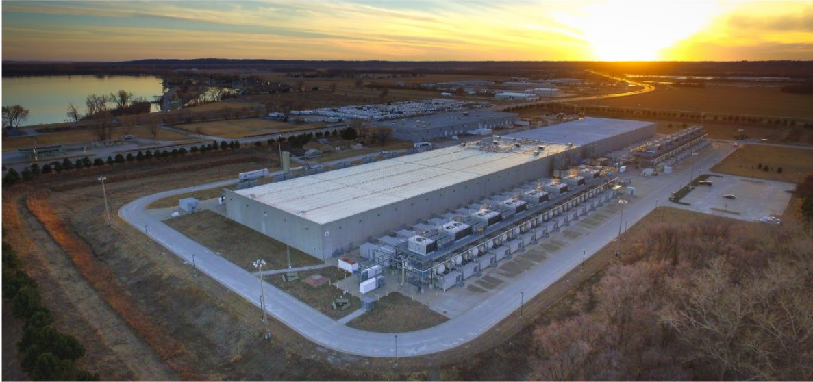
Google Data Center, Council Bluffs Iowa (49062863796).jpg from Wikimedia Commons by Chad Davis, CC-BY 2.0
