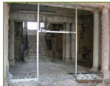
Figure 2-12: Deteriorated Grand Staircase (2017)
