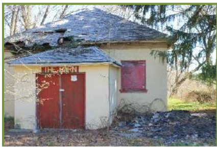
Figure 2-19: ‘The Barn’ Powerhouse
