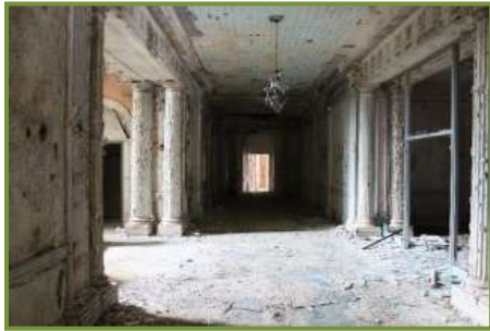
Figure 2-13: Water Damaged Grand Hall
