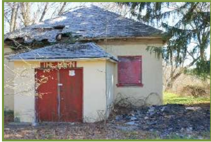
Figure ES-6: “The Barn” Power House
