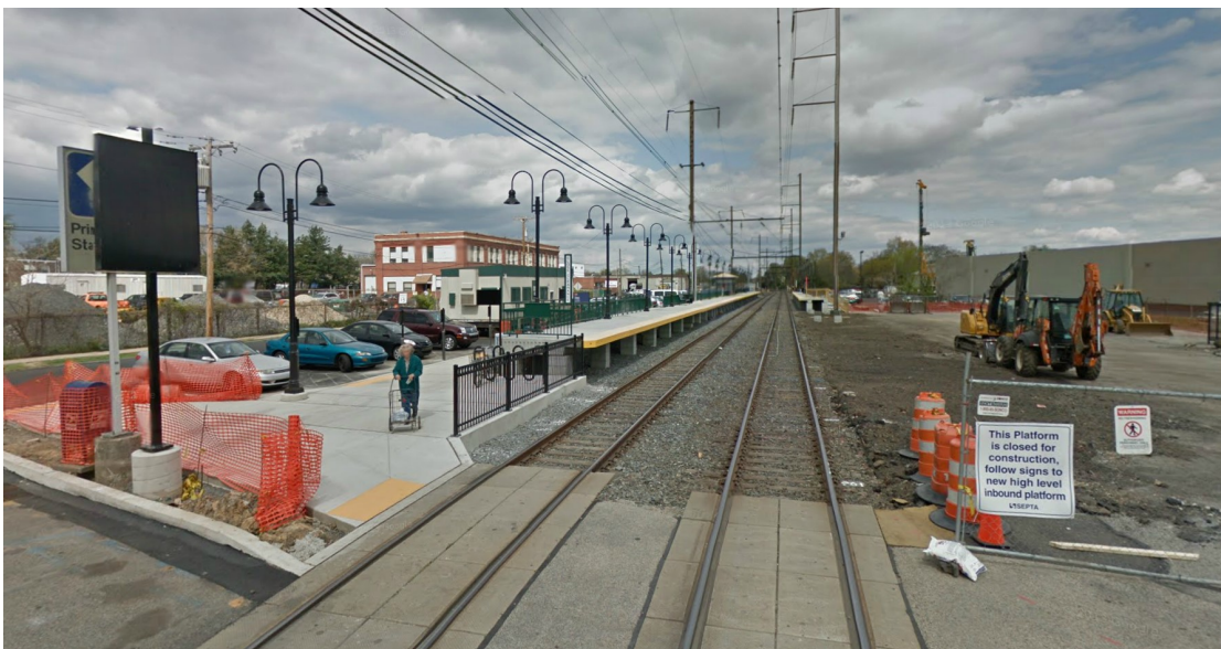
Construction of ADA accessible platforms at Primos Station on the Media-Elwyn Line. Image source: Google street view
