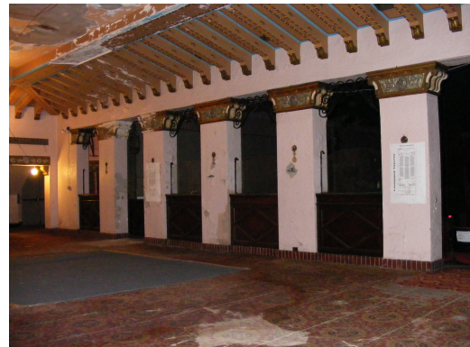
Capital Repair Needs Interior of Lansdowne Theater
