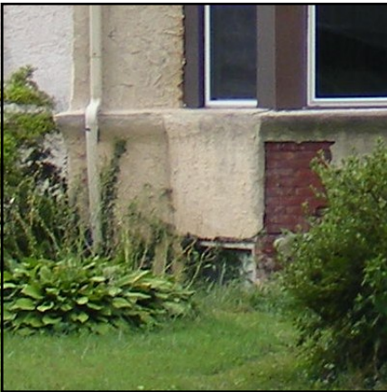
Modern cladding removed to expose moisture damage on original wall
