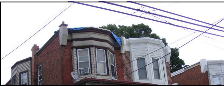
Note the original cornice and brackets on the left and the covered-up on the right.
