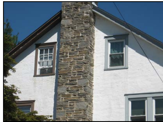
Note original multi-pane window on the left and inappropriate replacement on the right
