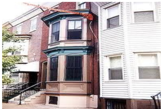
Note original dual pane windows on left and newer single pane windows on right
