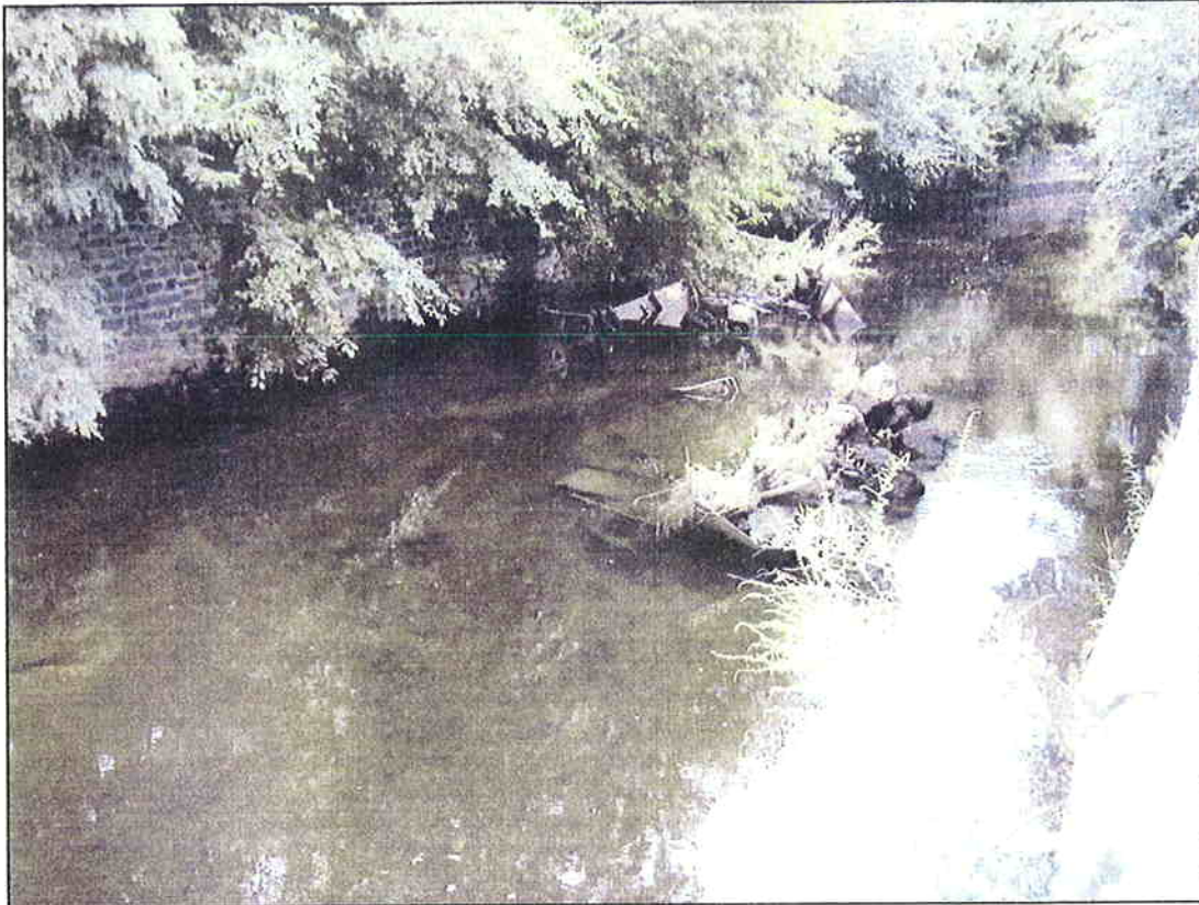
J-1, Baldwin Towers: shopping cart and silt in channel
