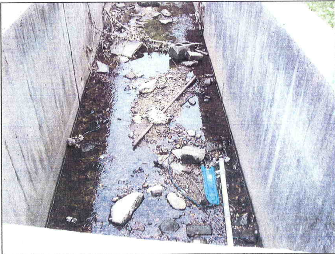
J-3, Walter St: heavy debris in channel
