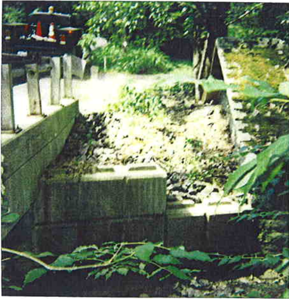
D15 - Topples @ Avondale Storm Drain Corp's Survey entering Dicks Run
