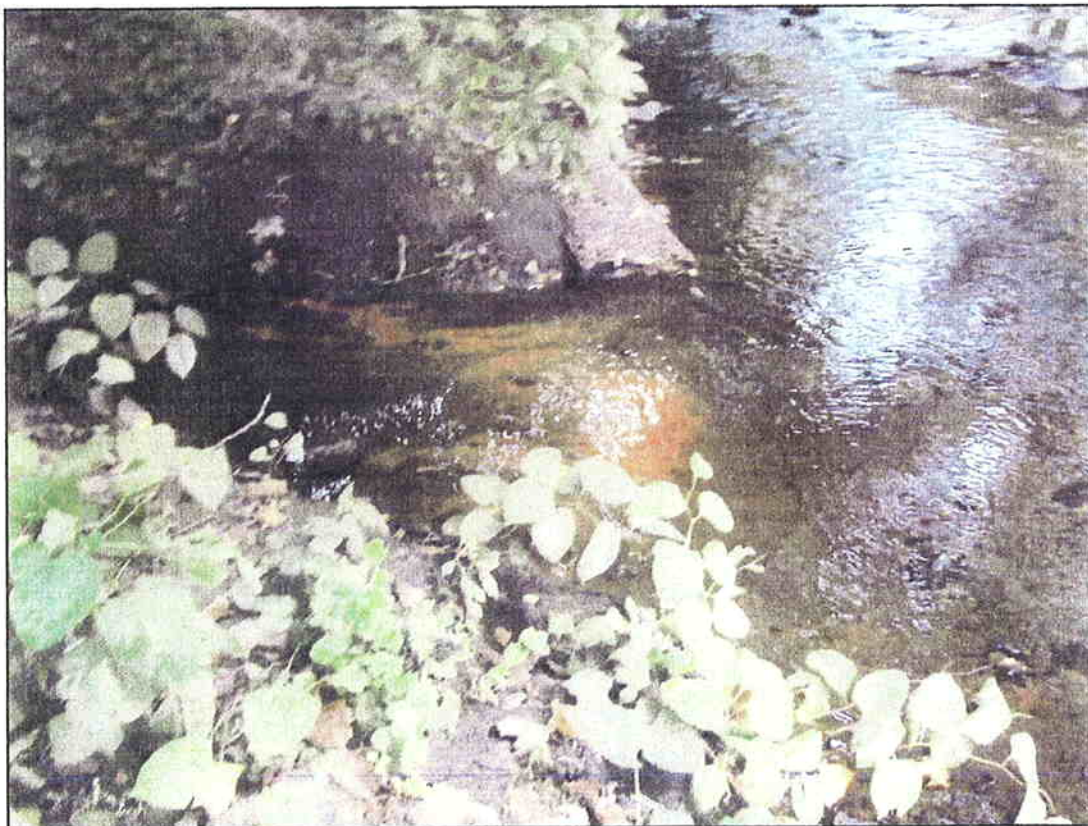
J-2, Chester Pike: orange deposits coming from outfall channel
