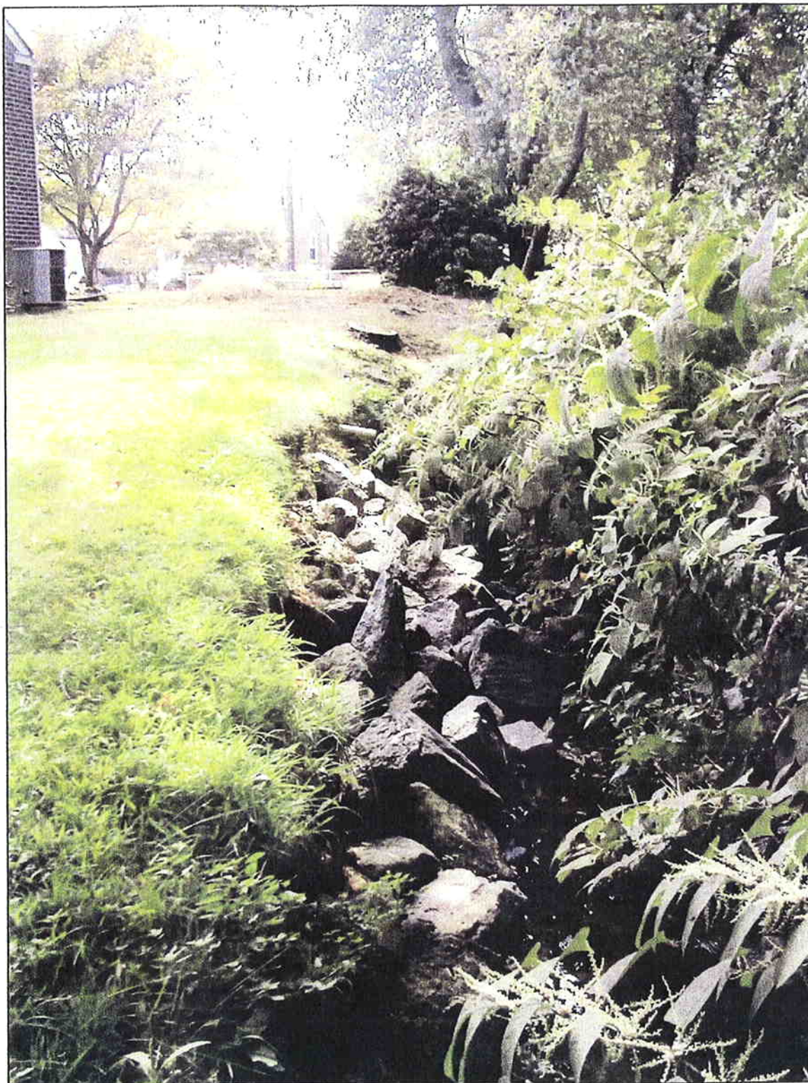
Little Crum Creek, Unnamed tributary Rip rap bank stabilization near Edgewood Ave and Village Rd Identified as A-12 and C-2
