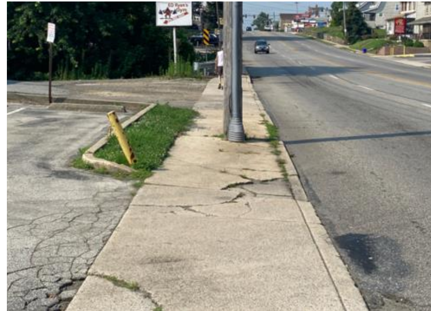
Figure 3-14: Utility pole narrowing the sidewalk at the intersection of South Avenue and Chester Pike
