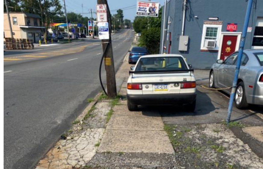
Figure 3-15: Blocked, damaged sidewalk outside of auto shop.
